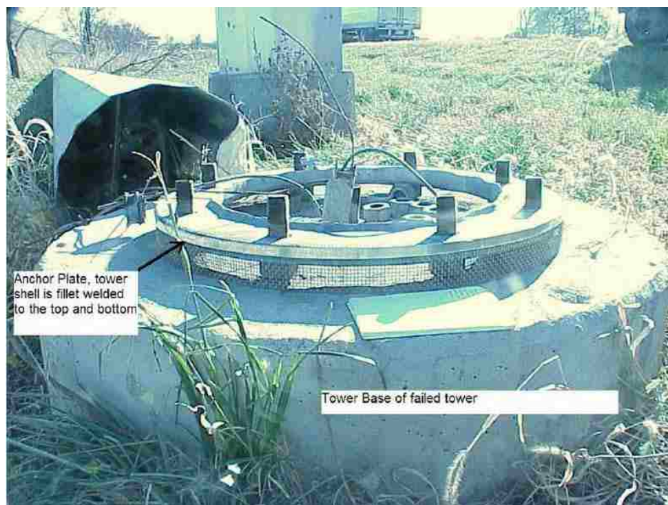
Figure 4. Close-up of collapsed tower ( reprinted from Dexter, 2004 )
