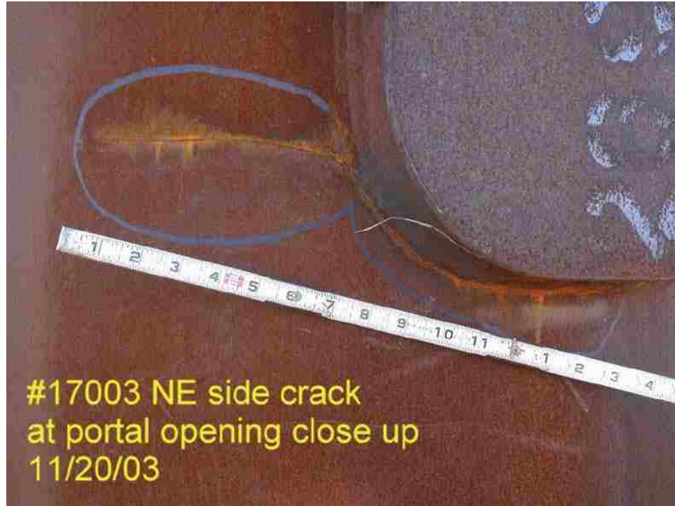
Figure 5. Handhole crack at corner ( reprinted from Koob, 2006 )
